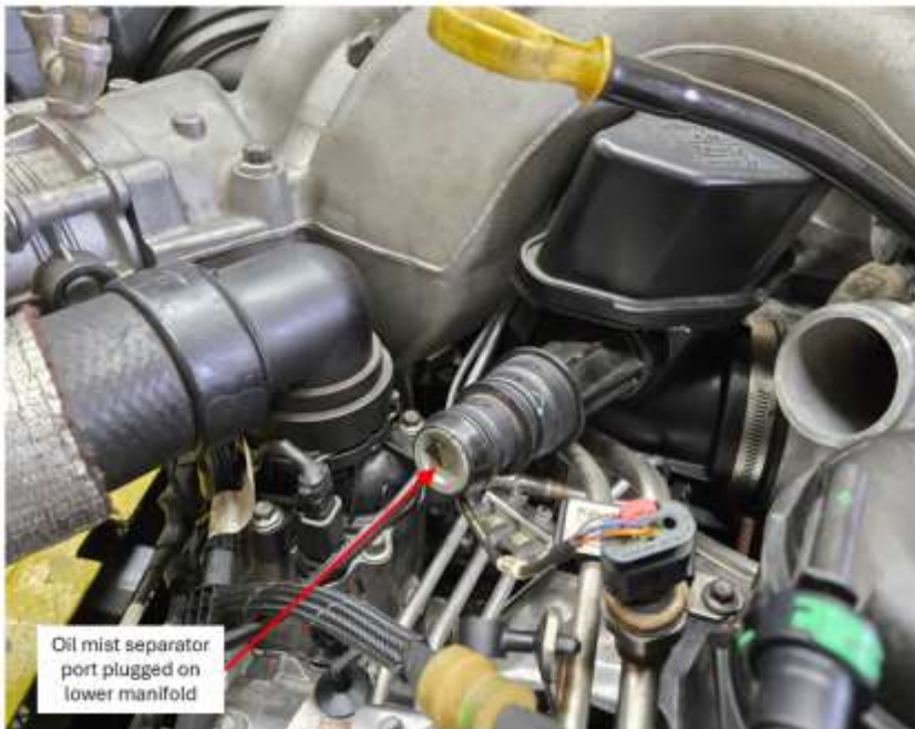
Figure A4.37 Oil Mist Separator Connection Port Blocked Off
